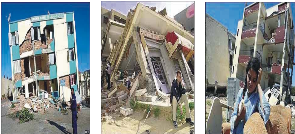
Figure 1.1: Failure of URM walls (Algeria 2003): a) In-plane Failure, b) Out-of-plane Failure, c) Combined Failure
