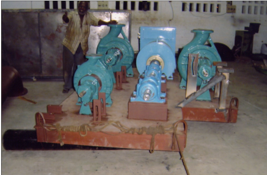
Figure B6.23 , The Assembled PAT System with Main Shaft (Ex-Workshop)
