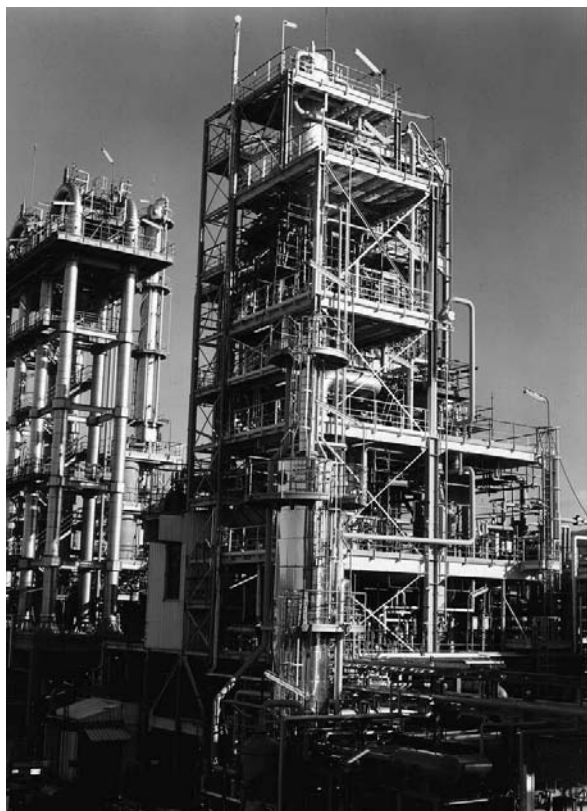
Fig. 1.11 : Production plant in chemical process engineering
