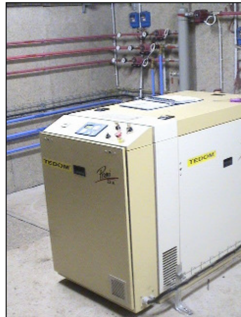
Figure 8: TEDOM CHP module
