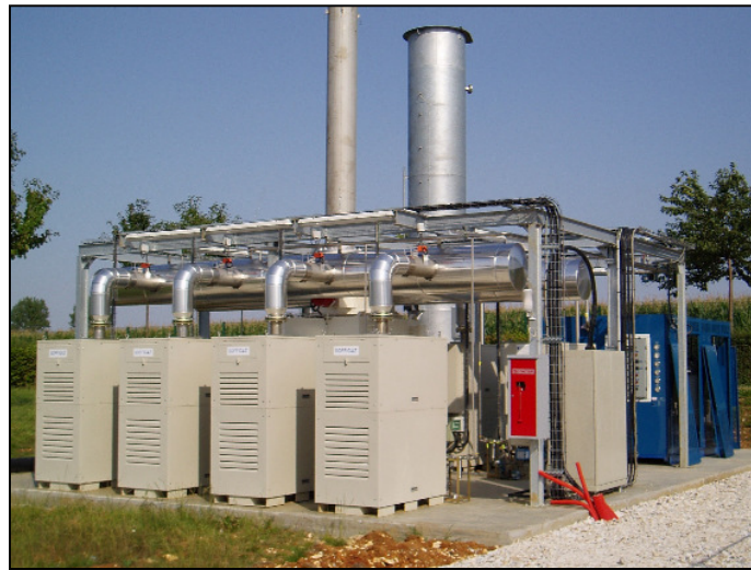
Figure 6: SMITOP's 8-microturbine plant
