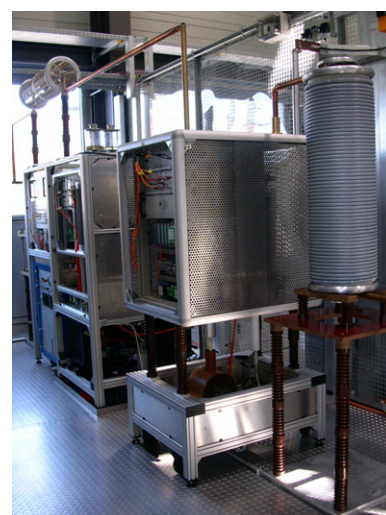
Fig. 4: Body power supply and crowbar / filament heating unit
