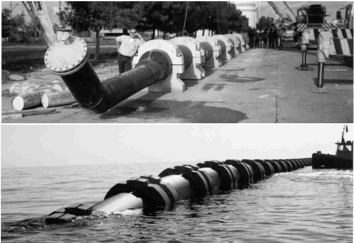
Fig. 10: Antalya outfall (Turkey) during installation in 1997. Top : Diffuser section assembling on shore. Down : Feeder section ( L_F = 5 \text{ km} , HDPE pipe, D = 1600 \text{ mm} ) while sinking with attached concrete weights on the seabed (PipeLife Company)
