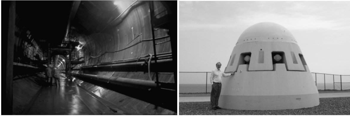
Fig. 11: Boston outfall during installation in 1998. Left: View into tunnel section (16 km with 8 m diameter). Right: One out of 55 riser caps with eight outlets each in rosette like configuration (Roberts and Snyder, 1993)
