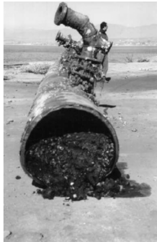
Fig. 16: Replaced diffuser, blocked with sediment (courtesy of Eng. Pedro Campos, Chile)
