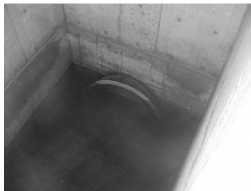
Fig. 25: Picture of the headworks of a coastal outfall showing the inlet to the feeder pipe (courtesy of Carlo Avanzini)
