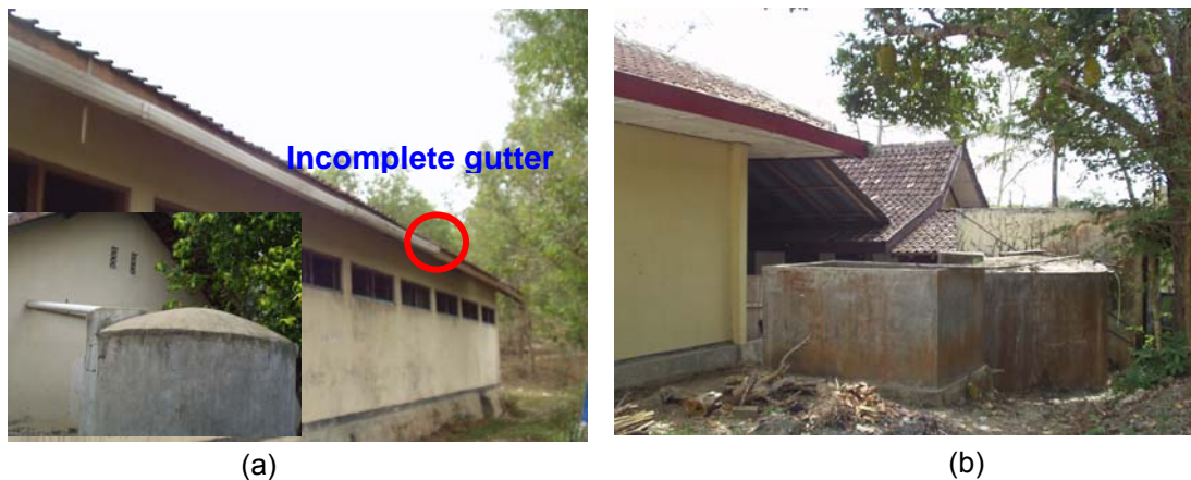
Figure 3.13: A failed RWH project was developed by the local Government in Prambanan: (a) The gutter for collecting rainwater is insufficient, and the water storage originally for storing rainwater is dominantly used for collecting water from the Government. (b) Rainwater storage is also abandoned by people who prefer to get water from the Government. (Photo: Widodo, 2005)
