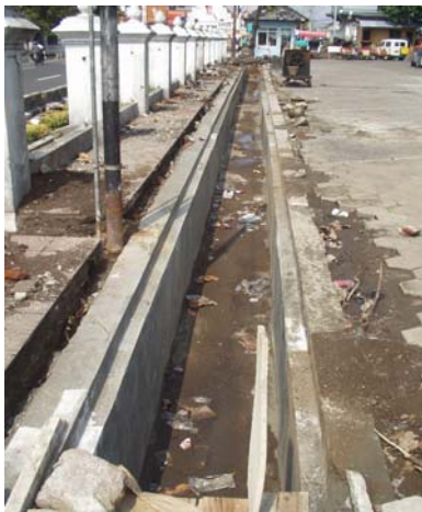
Figure 2.10: Rainwater drainage system was being developed in Malioboro area, Yogyakarta. The rainwater is drained into Code River directly. There is no rainwater infiltrating into the ground. This system indicates the conventional paradigm of drainage system in Yogyakarta and other places (Photo: Widodo, 2004)
