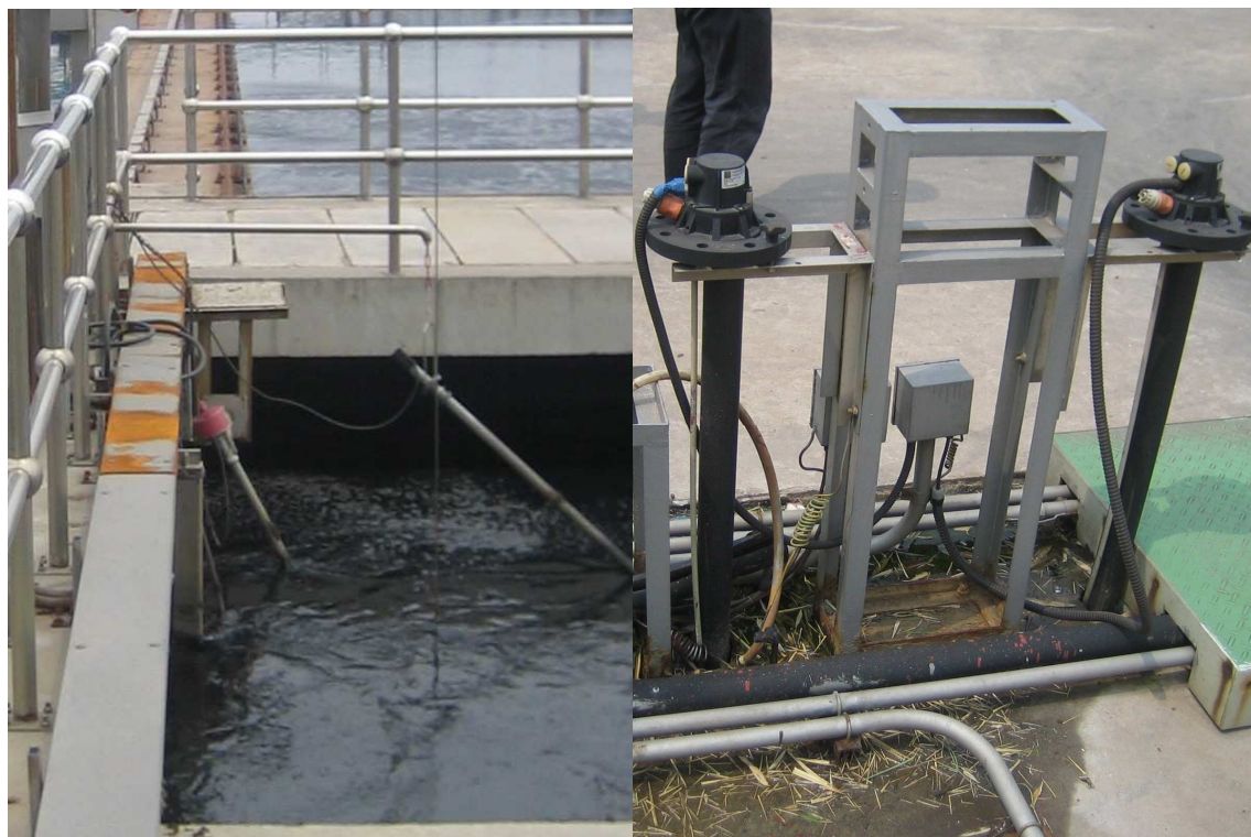
FIGURE 121: SENSORS FOR ONLINE MEASUREMENT IN CHINA
