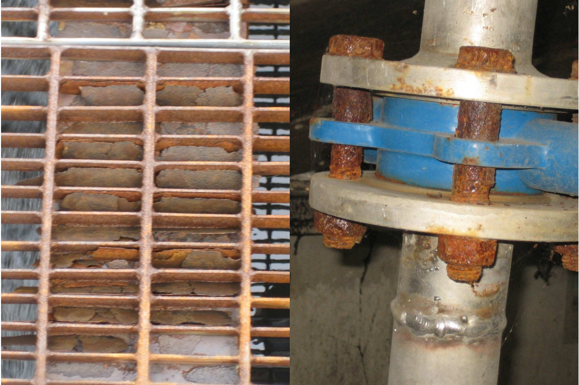
FIGURE 100: CORROSION ON GALVANISED COVERS AND BOLT CONNECTIONS IN CHINA
