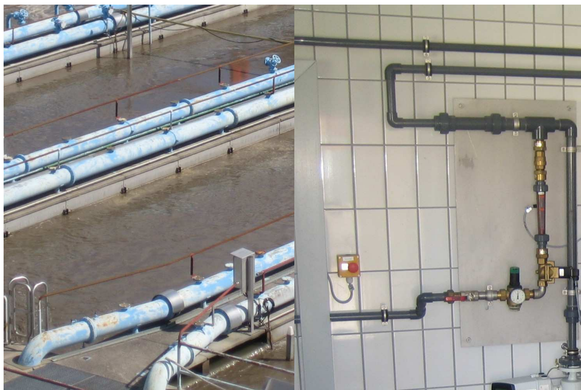
FIGURE 155: PIPING AND MOUNTINGS ON STPS IN GERMANY
