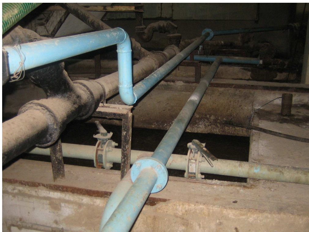
FIGURE 47: UNORGANISED AND UNSTABLE PIPING IN INDIA
