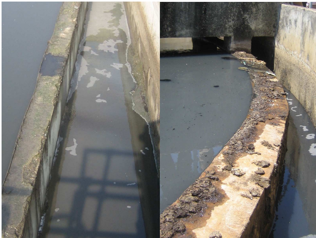
FIGURE 45: FLAKING AND DIRT ON CONCRETE WEIR EDGES ON STPS IN INDIA
