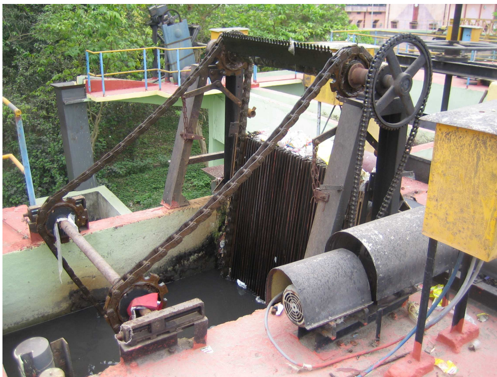
FIGURE 58: AUTOMATIC BAR SCREEN IN INDIA
