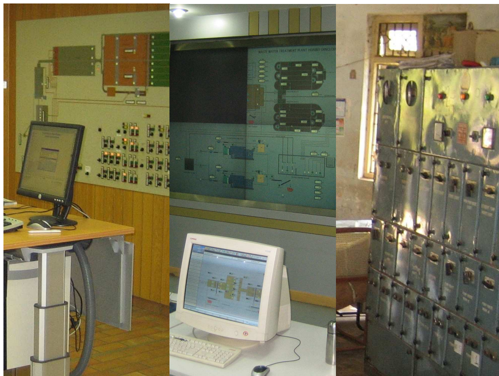
FIGURE 196: CONTROL ROOMS IN GERMANY (LEFT), CHINA (MIDDLE) AND INDIA (RIGHT)
