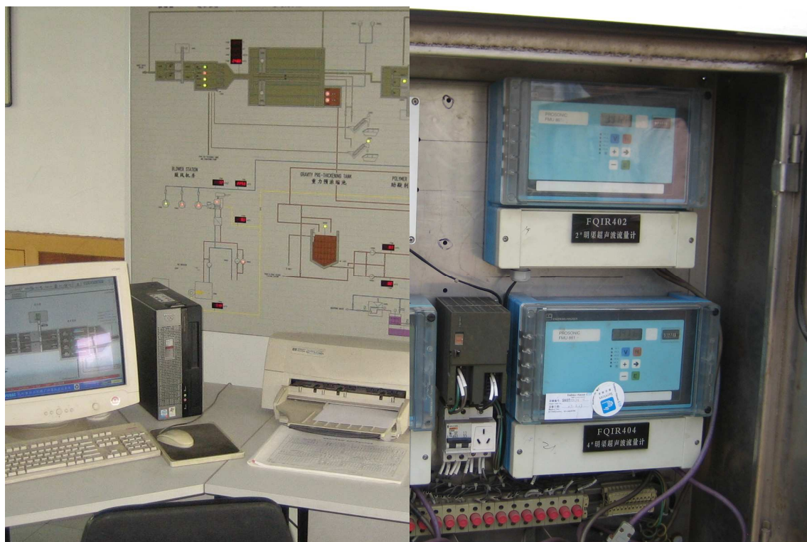
FIGURE 122: CENTRAL CONTROL ROOM AND OUTDOOR CONTROL PANEL IN CHINA
