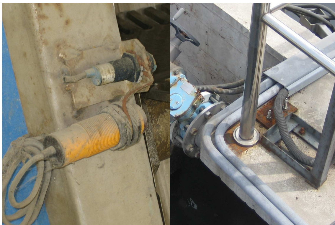
FIGURE 119: CABLING ON STPS IN CHINA
