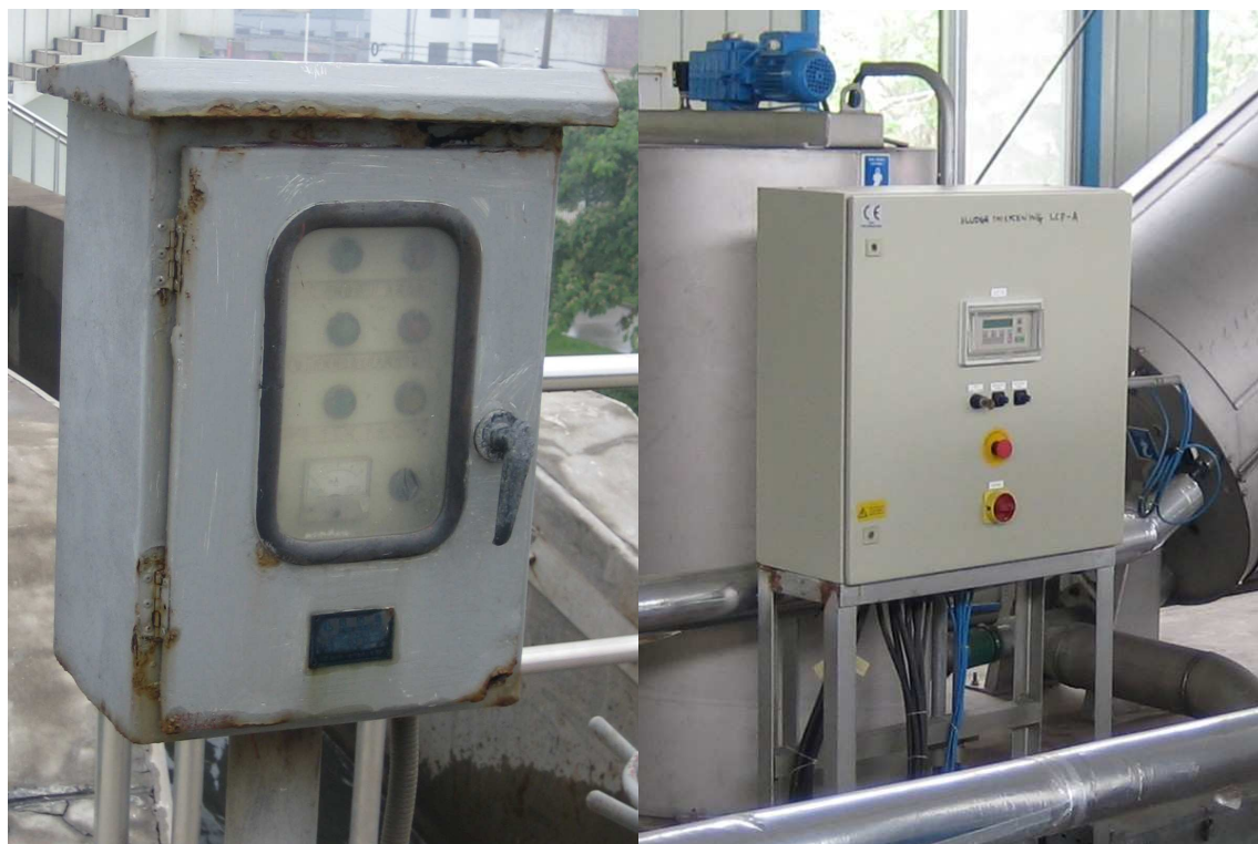
FIGURE 120: OUTDOOR AND INDOOR CONTROL PANELS ON STPS IN CHINA
