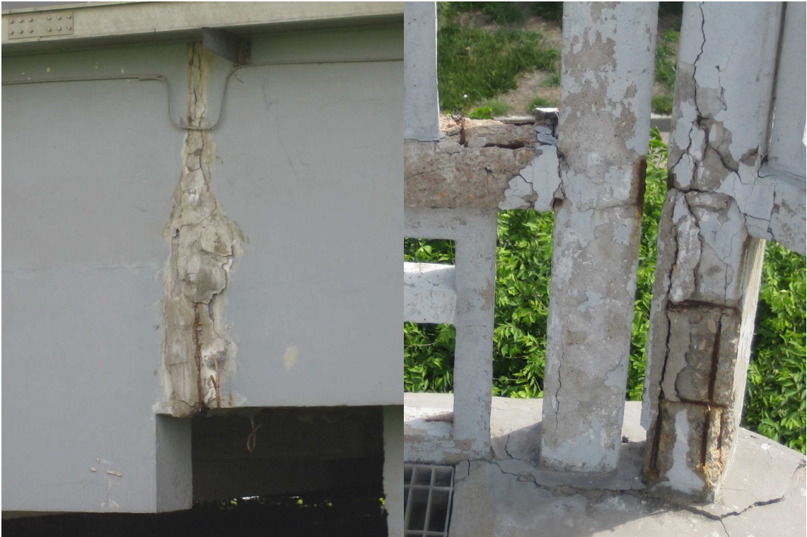
FIGURE 99: FISSURES AND FLAKINGS OF CONCRETE STRUCTURES IN CHINA
