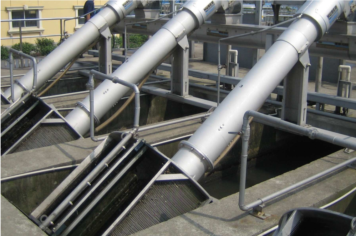
FIGURE 110: GERMAN STAINLESS STEEL SCREENING SYSTEMS IN CHINA
