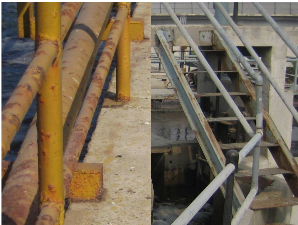
FIGURE 46: CORRODED HANDRAILS AND MOUNTINGS ON STPS IN INDIA
