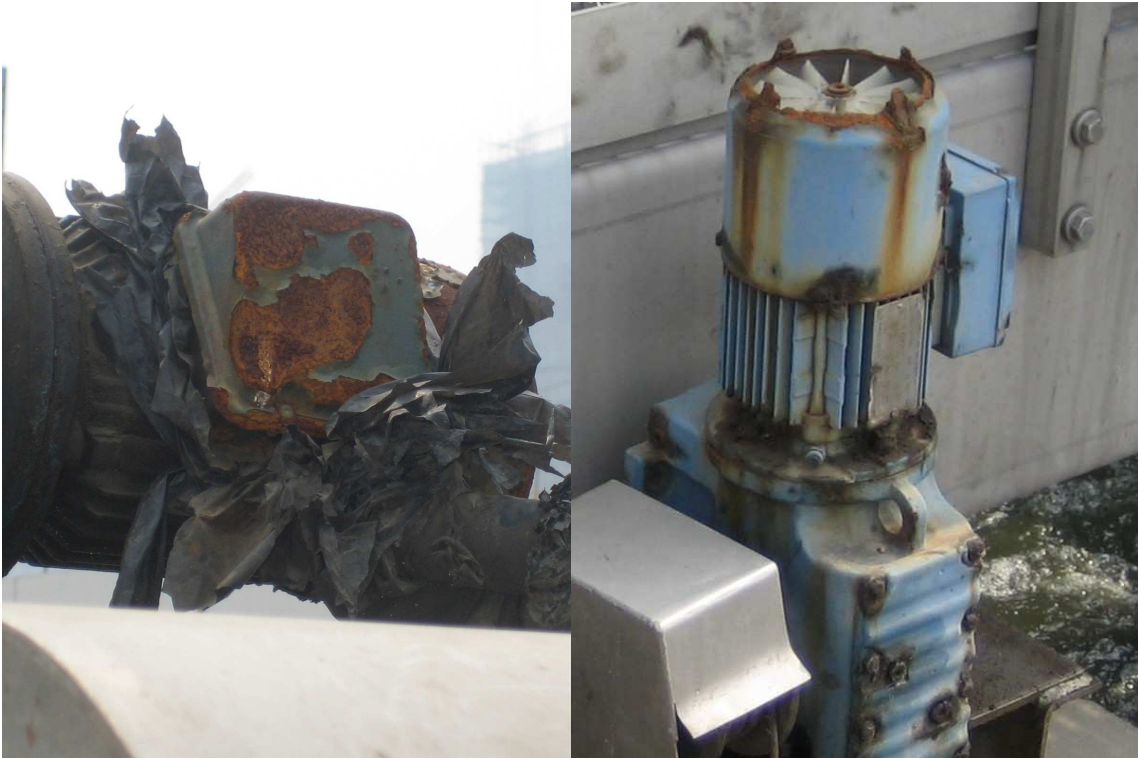
FIGURE 109: CORRODED DRIVE COMPONENTS IN CHINA
