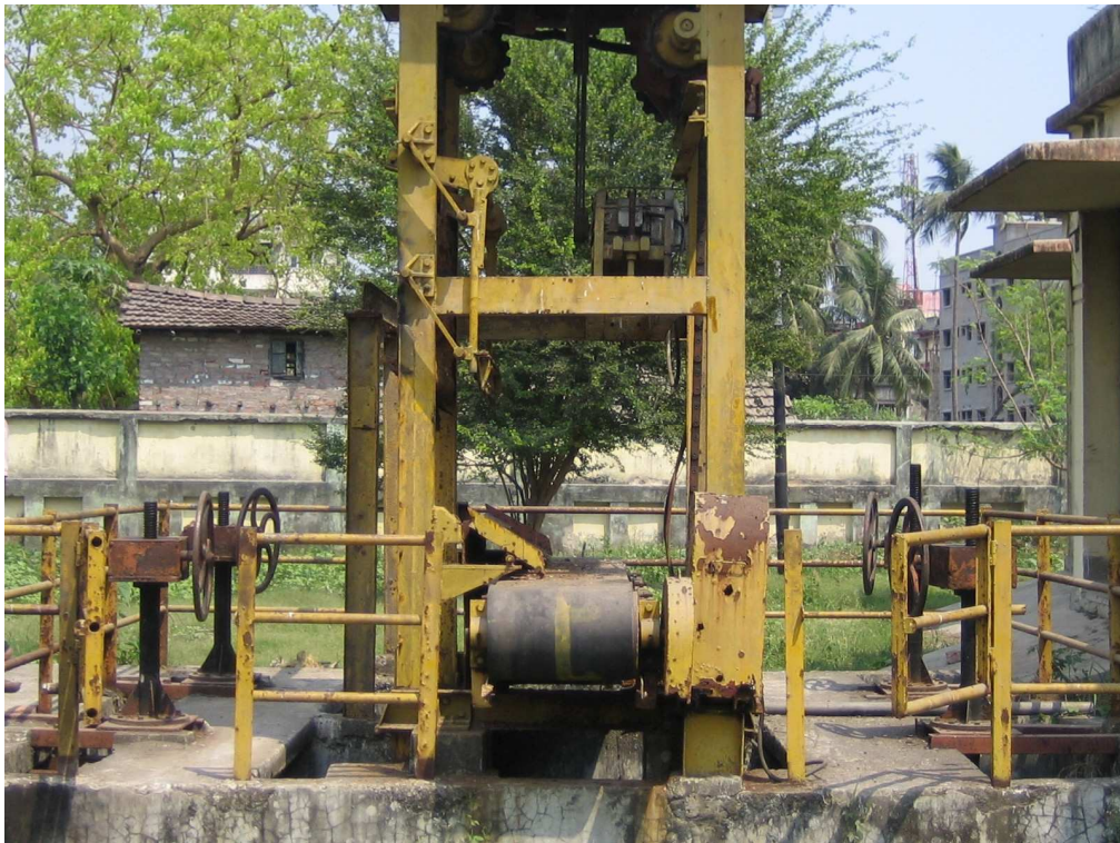
FIGURE 55: SEVERELY CORRODED FINE SCREEN IN INDIA
