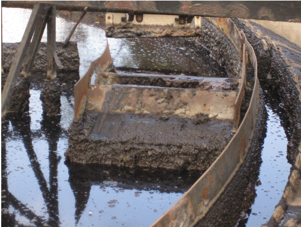
FIGURE 54: DIRT COVERED AND SEVERELY CORRODED SCRAPER BRIDGE AND WEIR EDGE IN INDIA
