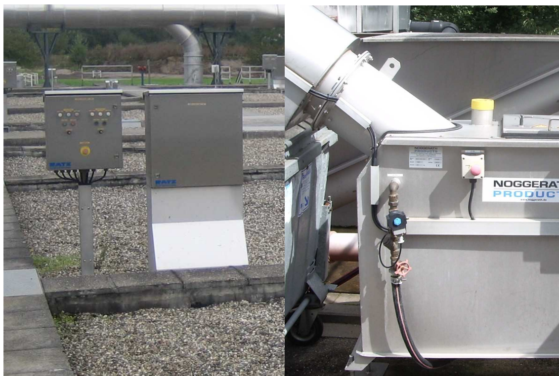
FIGURE 170: OUTDOOR CONTROL PANELS AND CABLING IN GERMANY
