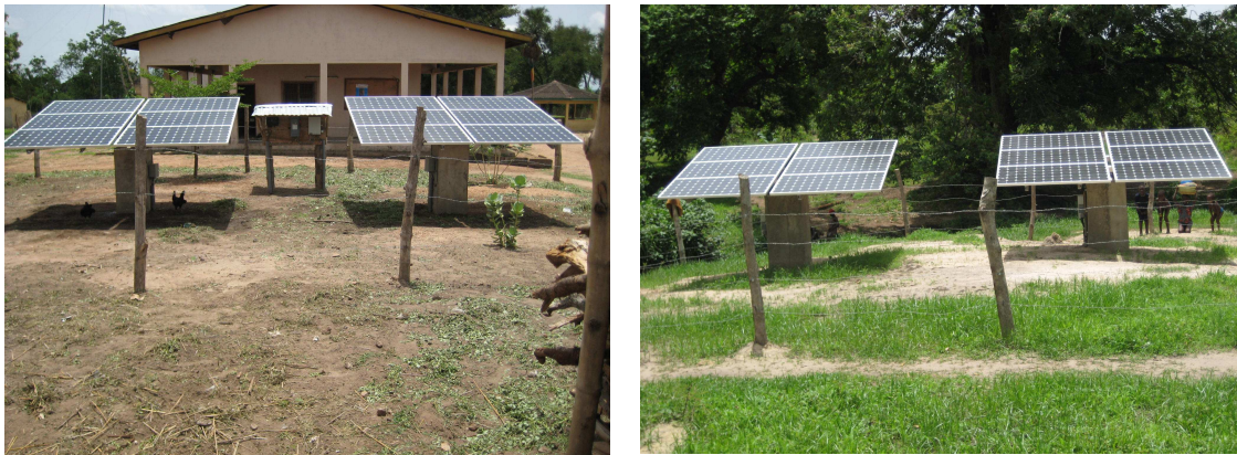
Photo 6: PV arrays in Dunkassa and Bessassi in Kalala – Benin (Photo: Noumon, 2008)
