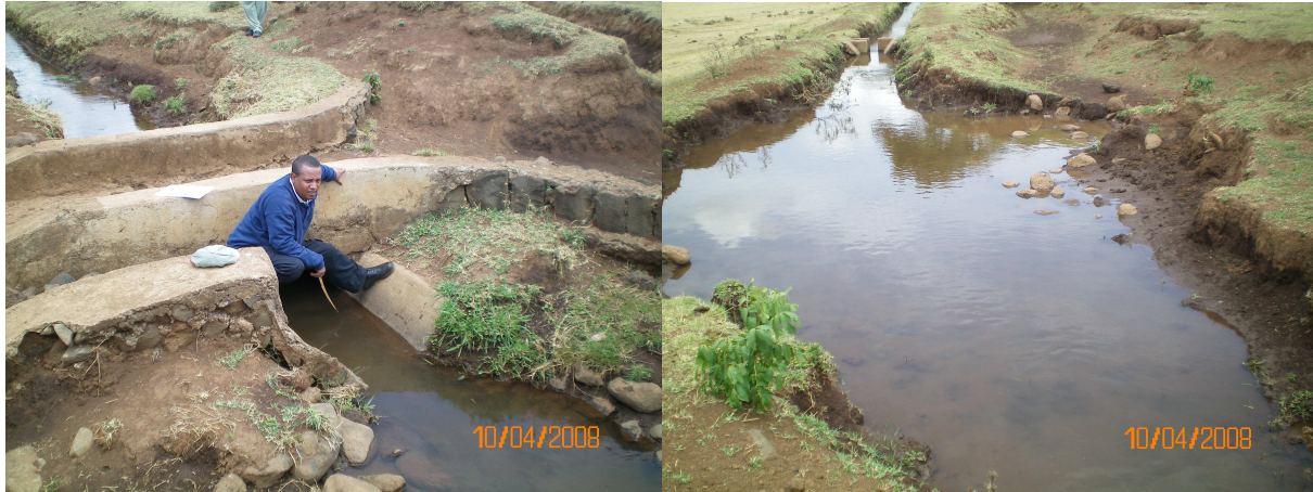
Figure 36 Canal breaching along the main canal for Kulanti irrigation project
