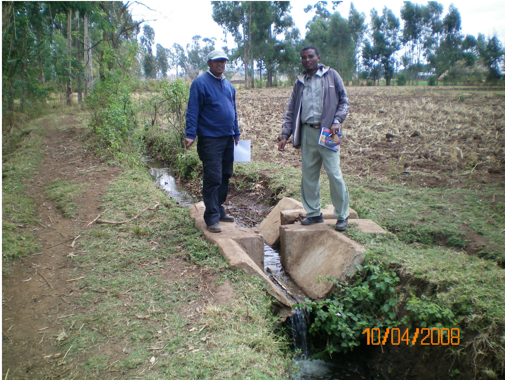
Figure 5 Effect of a scoured drop structure on the canal full supply level
