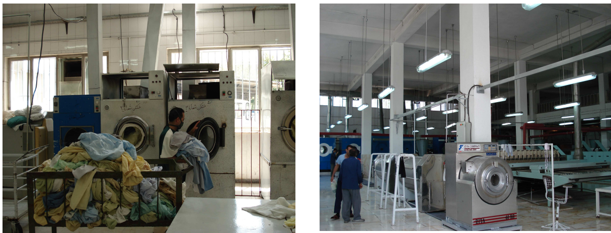
Figure 4-11: View in the laundry (Iran)
