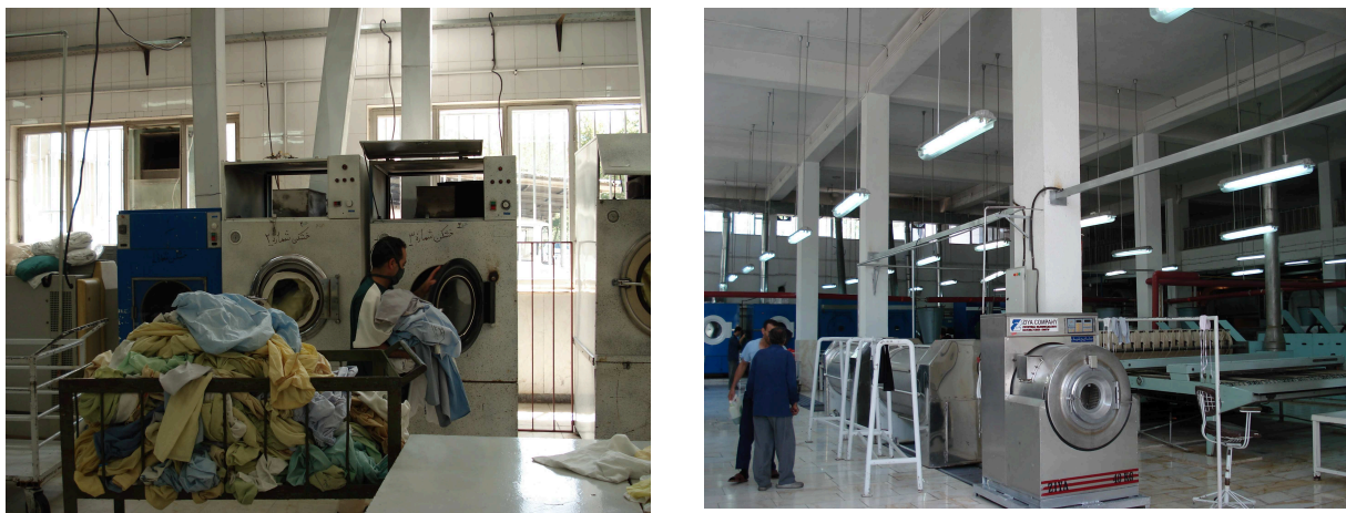
Figure 4-11: View in the laundry (Iran)
