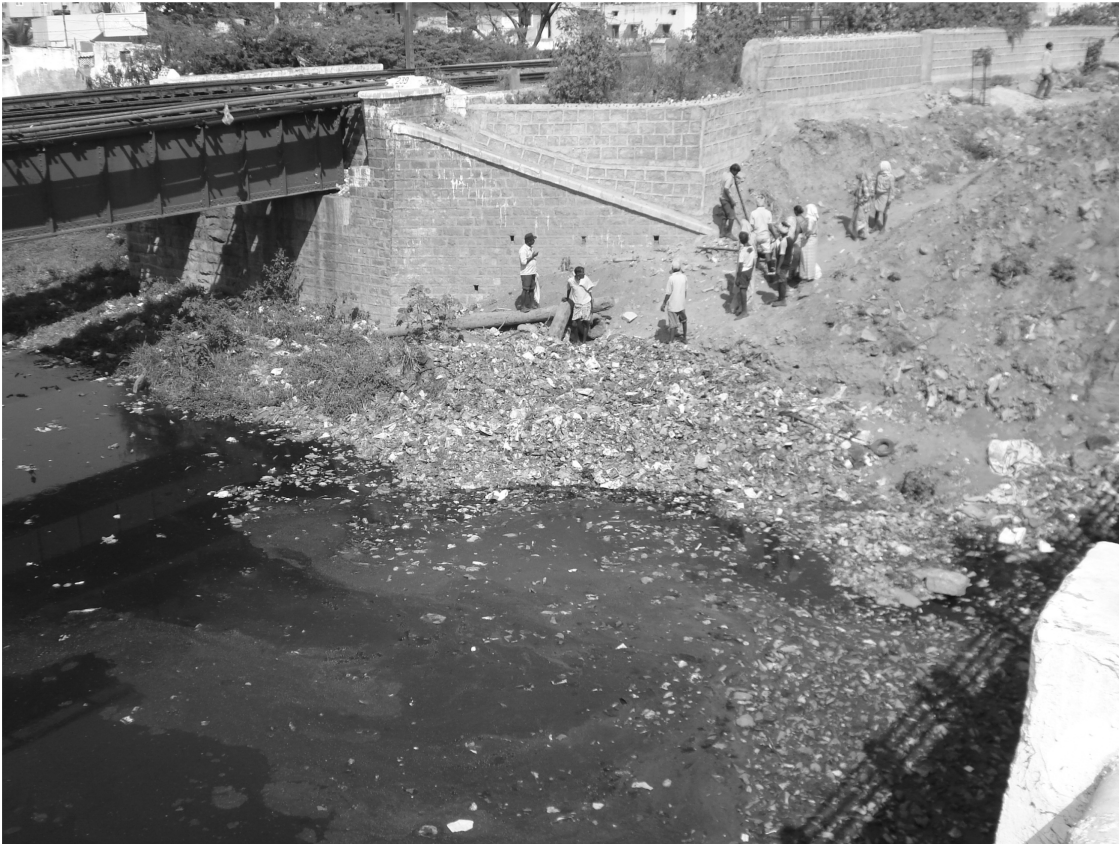
Figure 2.6: Sewage inflows in one of the inlets of Hussain Sagar lake, Hyderabad (Source: CRE, Hyderabad)
