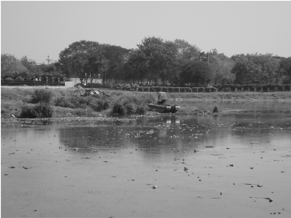
Figure 2.7 Dredging being carried out in Hussain Sagar Lake, Hyderabad (Source: CRE, Hyderabad)
