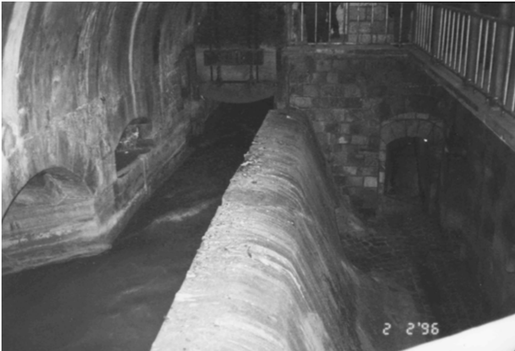
Fig. 4: Overflow structure in the sewer network of Vienna (Austria). If the combined wastewater sewer on the left side of the picture is brim-full with the mixture of sewage and stormwater the excessive volume gets discharged directly to the Danube river by overflowing the dividing wall in the middle of the picture. The residues on the wall coping show that it is waste water which gets discharged and not rain water, even though this phenomenon is often called "stormwater overflow" in the literature. [Photo: H. Lehn 1996]
