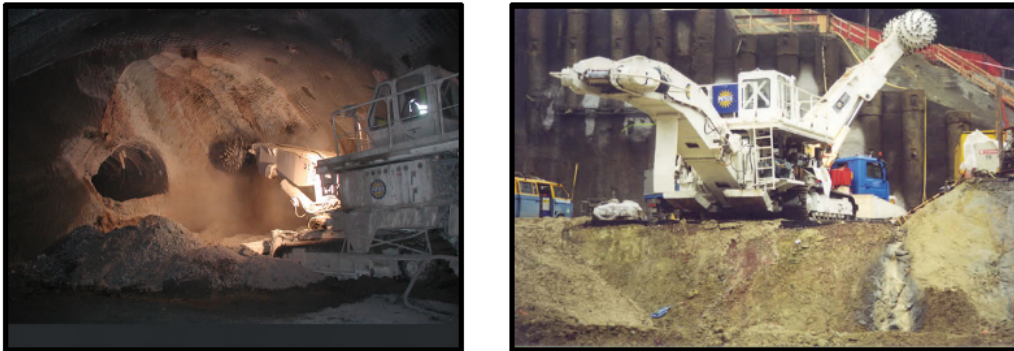
Figure 1.4.: Roadheading machine inside and outside a tunnel construction site (taken from www.pitsch.ch , 2009).
