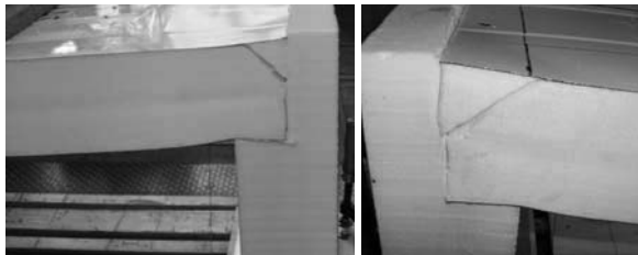
Figure 11: Failure of glued corner details
