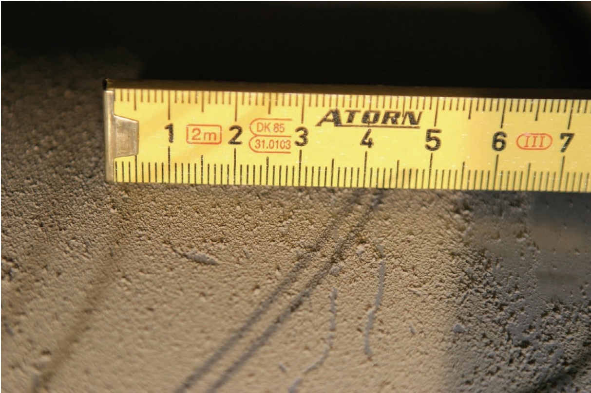
Fig. 4-26. KH01: Melt particles at containment wall
