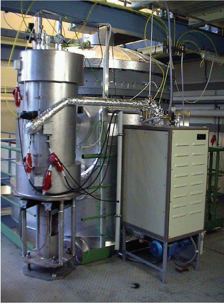
Fig. 3-23. The steam accumulator (left) and the steam generator (right)
