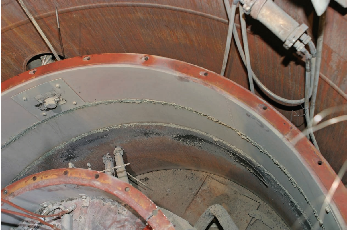
Fig. 4-19. KH01: Post test view of subcompartment 1
