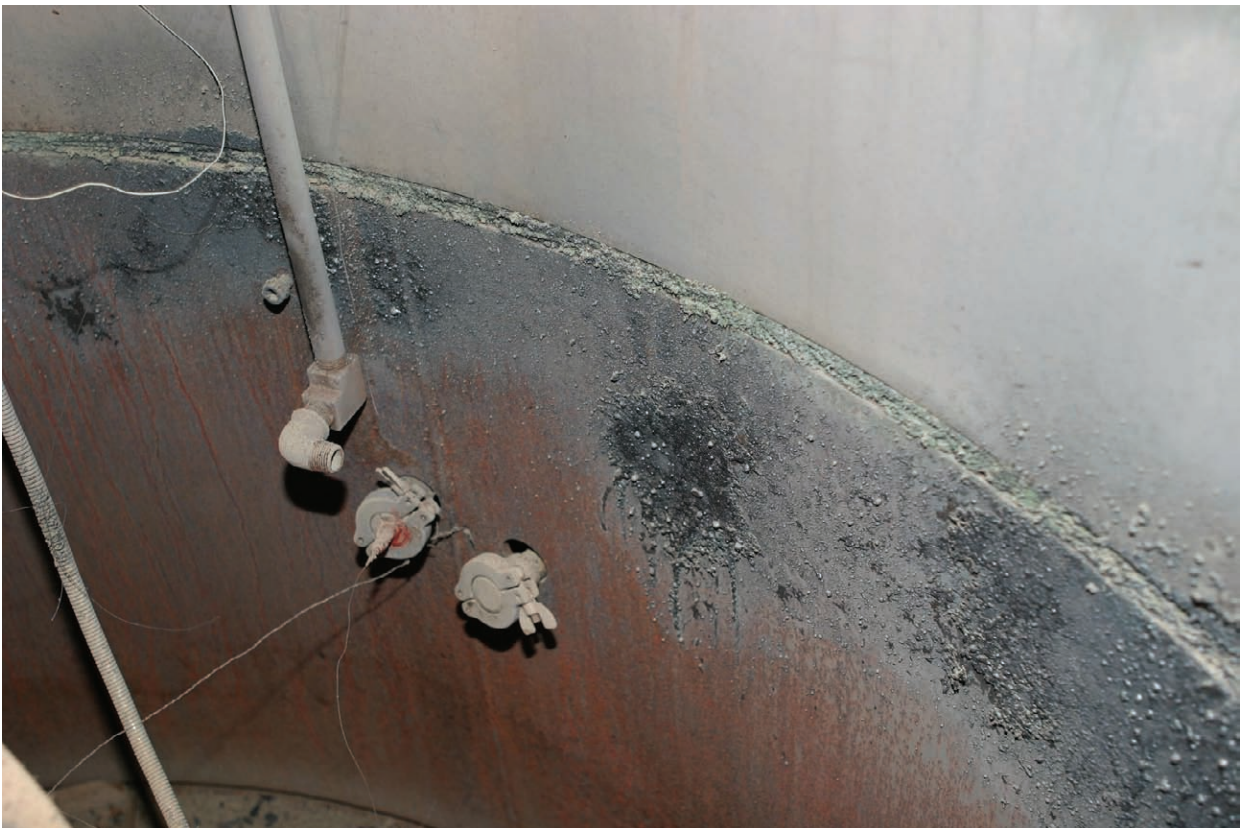
Fig. 4-20. KH01: Post test view of subcompartment 1 wall
