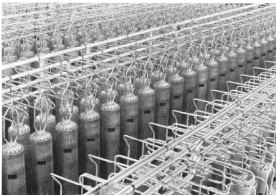
Figure 8.2.1. Centrifuge cascade hall of a gas centrifuge enrichment plant (URANIT).
