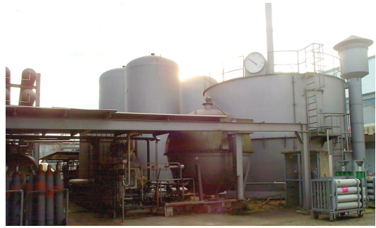
Fig. 3: Helium storage system.
