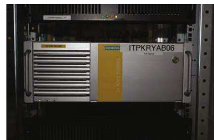
Fig. 6: New PCS7 Engineering station.
