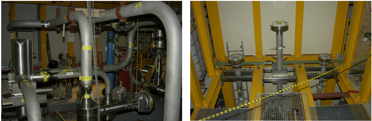
Fig. 1: Left: HELOKA construction site (hot side piping); right: test section connecting flanges.
