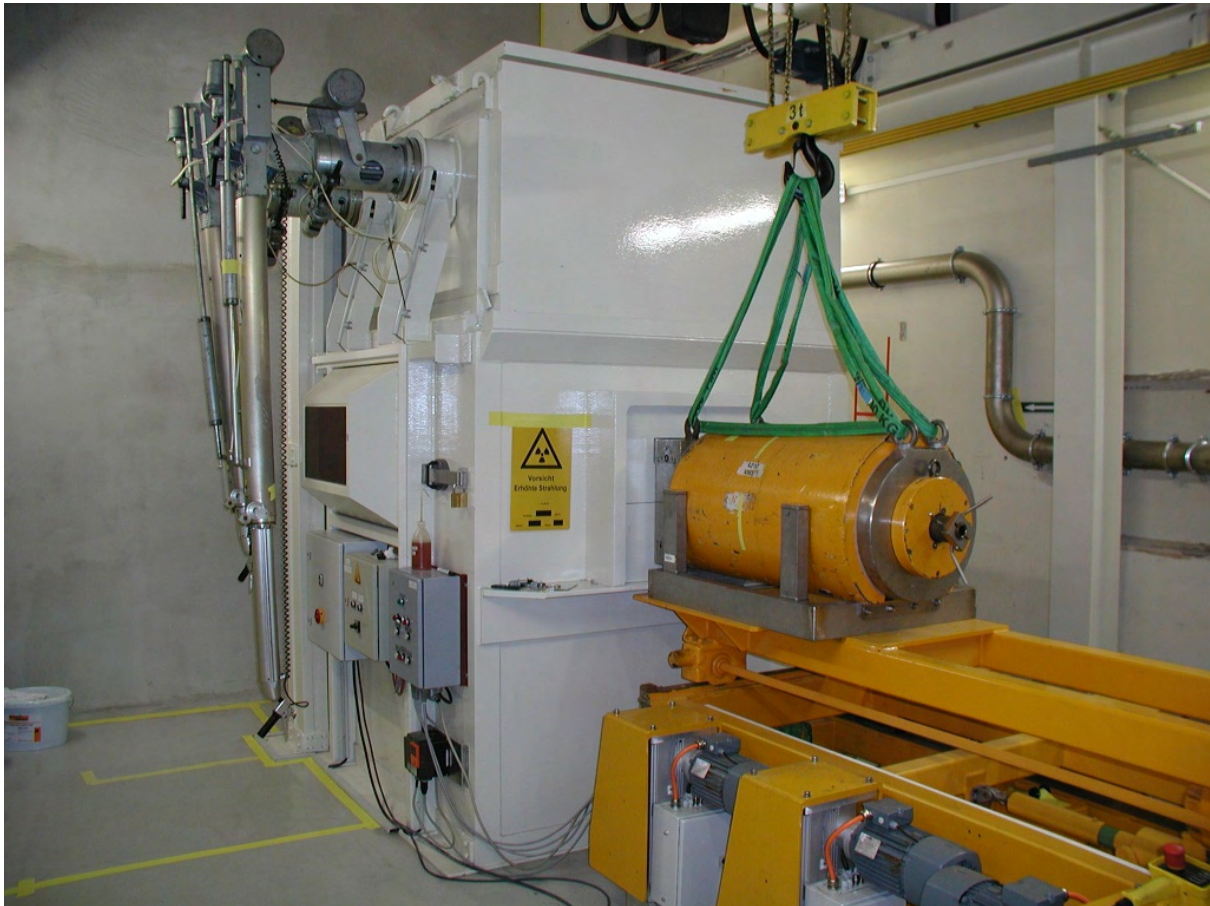
Fig. 1: Newly installed shielded transfer cell with positioning and docking system for various transport casks.
