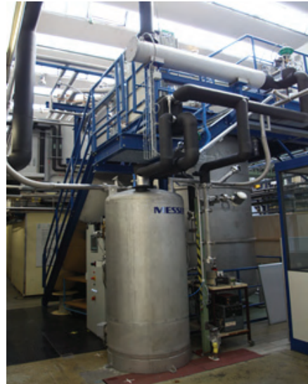
TIMO-2 facility: New 100 K supply facility
