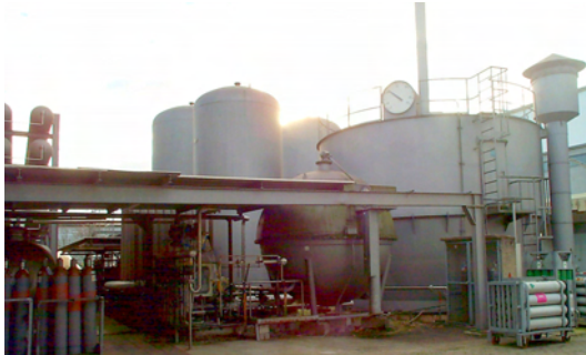
Fig. 3: Helium storage system.
