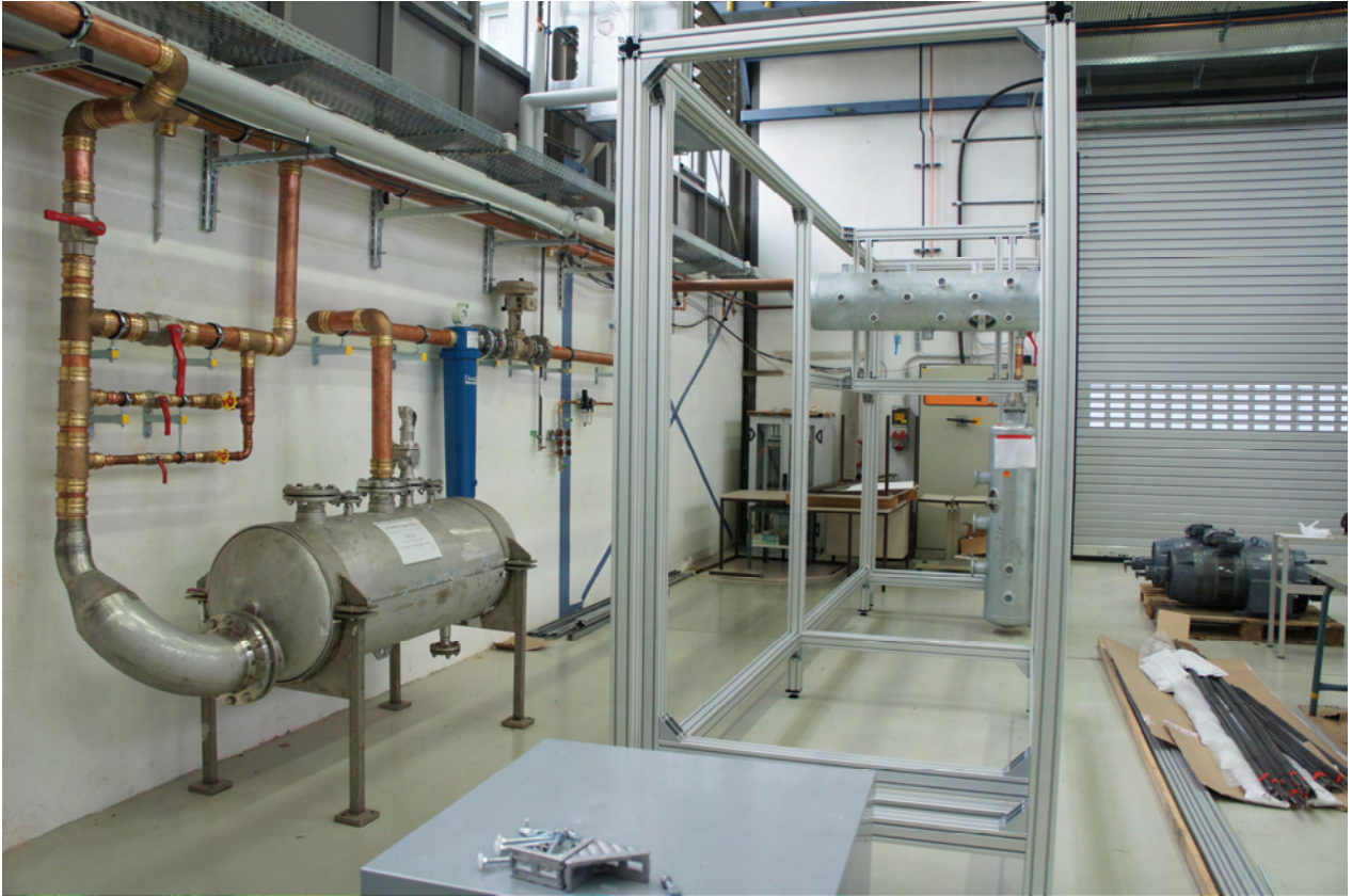
Fig. 4: Main supply line of pressurized air for Gricaman facility.
