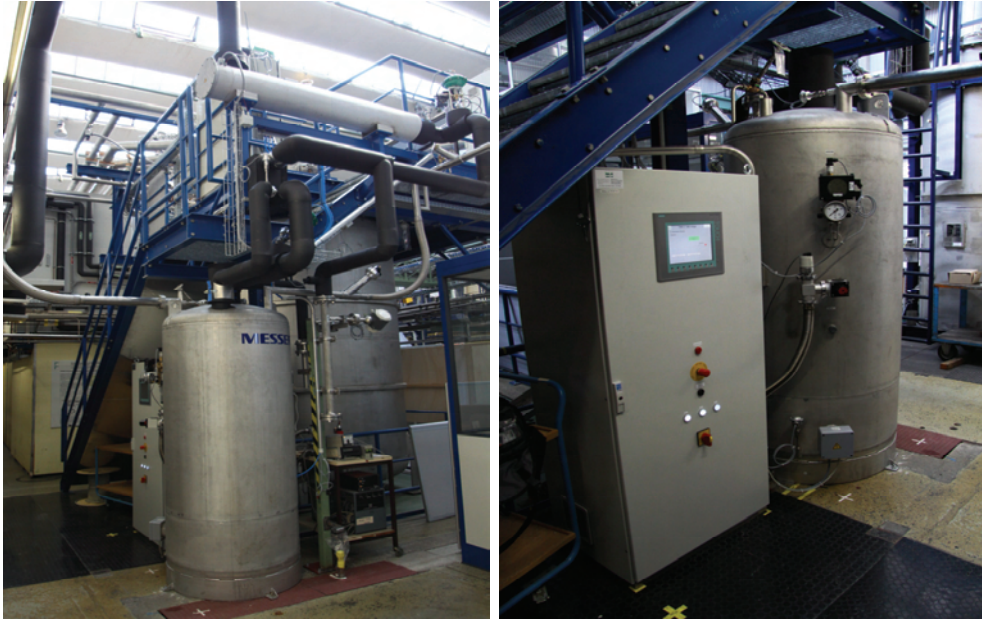
Fig. 3: The new 100 K facility integrated in the TIMO-2 cryogenic supply system.
