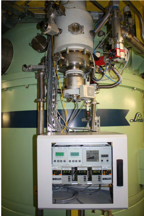
Fig. 5: New turbo molecular pumps including control system for cold and valve box.
