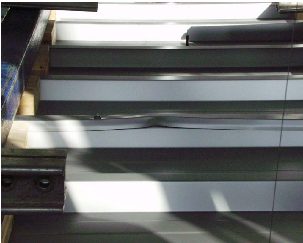
Fig. 9: Buckling of the overlapping unsupported edge
