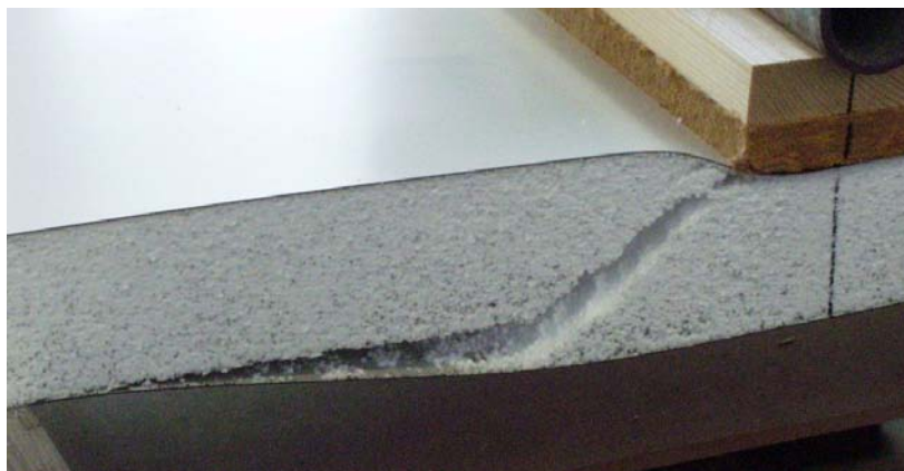
Fig. 2.4: Shear failure of the core
