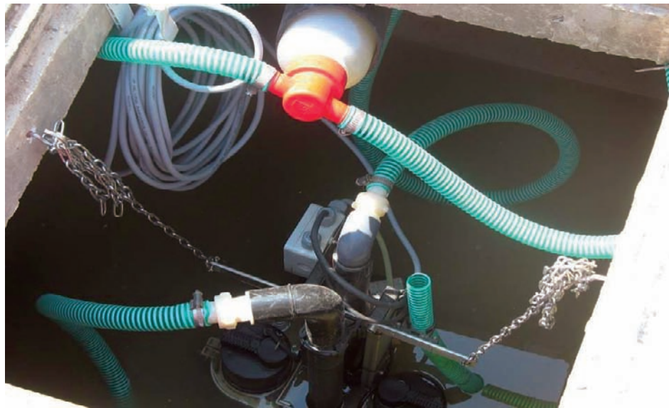
Figure 5.5 SBR unit under operation at the Fuheis test site, Jordan
