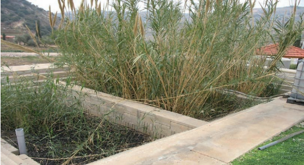
Figure 5.13 Sludge drying beds under sludge operations at Fuheis site
