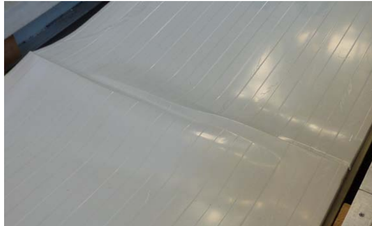
Fig. 4.2: Wrinkling in mid-span
