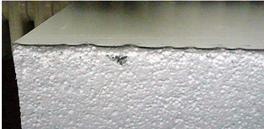
Fig. 4.7: Cracks between core and face and uneven cut edge
