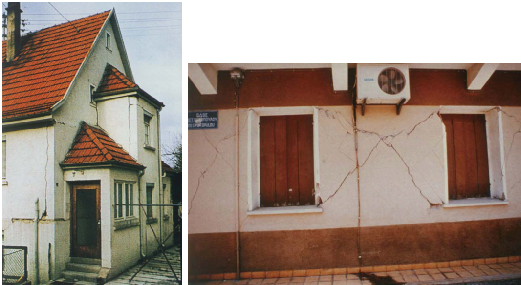
Figure 42: Exemplified earthquake induced building damages of category 2 (left) (1978, Albstadt, Germany) and 3 (right) (1995, North Peloponnissos, Greece) (Grünthal (1998), p.73, p.77)
