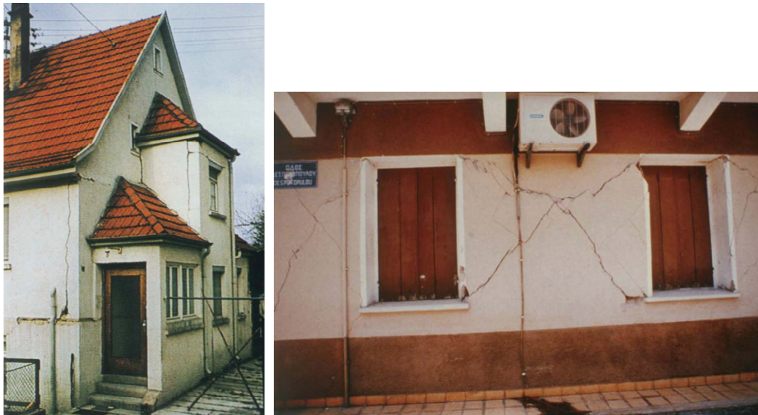
Figure 42: Exemplified earthquake induced building damages of category 2 (left) (1978, Albstadt, Germany) and 3 (right) (1995, North Peloponnissos, Greece) (Grünthal (1998), p.73, p.77)
