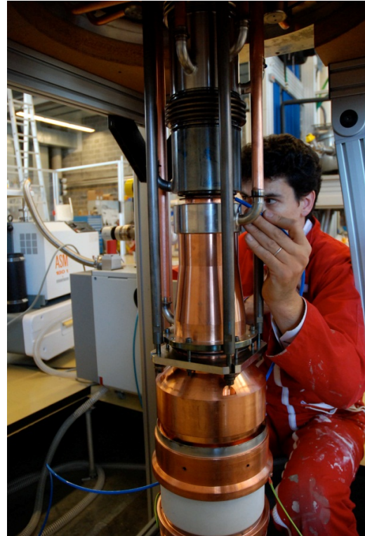
C. Lievin (TED) fixing the vacuum leak.
