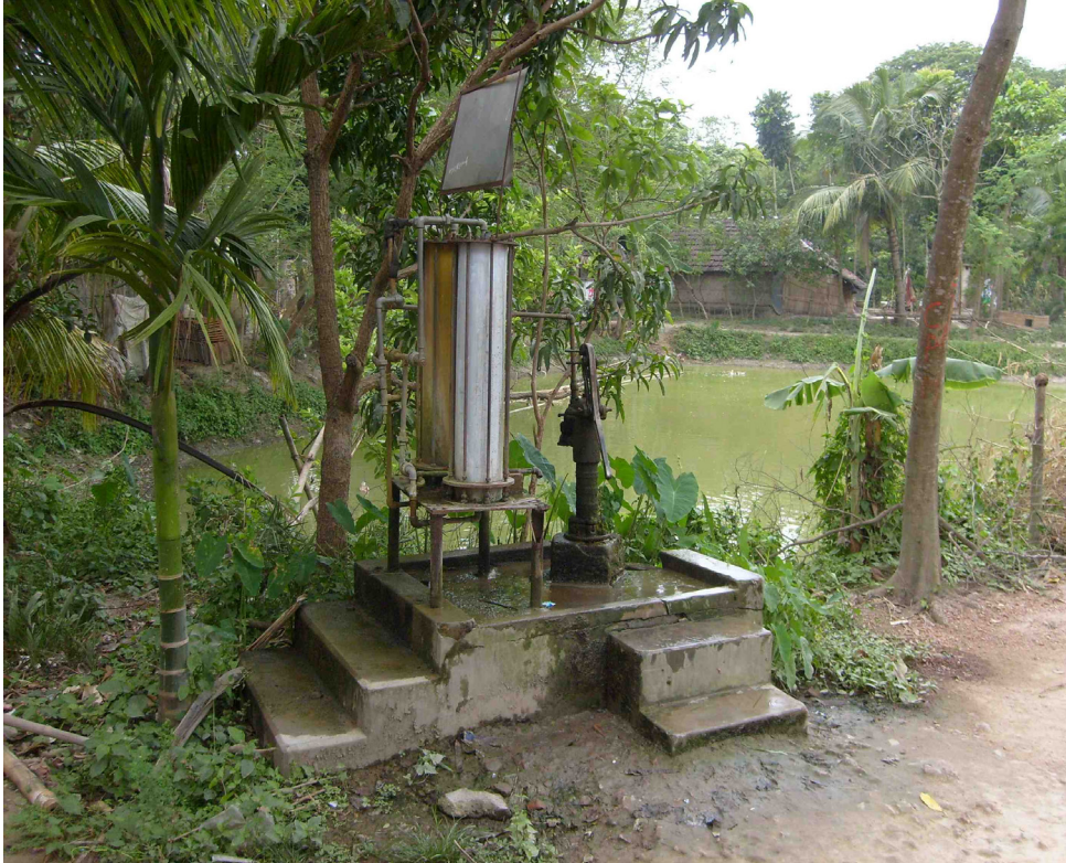
Figure 5.4: Picture of a public well installed in 2003 in the village Chakudanga, which is equipped with an As filter cartridge (well depth: 163 m). Surprisingly, the As concentration in filtered water was higher as compared to the raw water ( 77.4 compared to 101 \mu\text{g L}^{-1} ), strongly suggesting that the filter material needs to be replaced. This example demonstrates that current mitigation strategies (use of deep wells and filter systems) can be unreliable.
