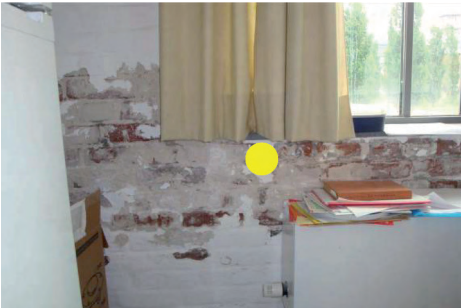
Figure 6: Interior wall, damage on the finishing layer. The sampling place is marked in yellow.
