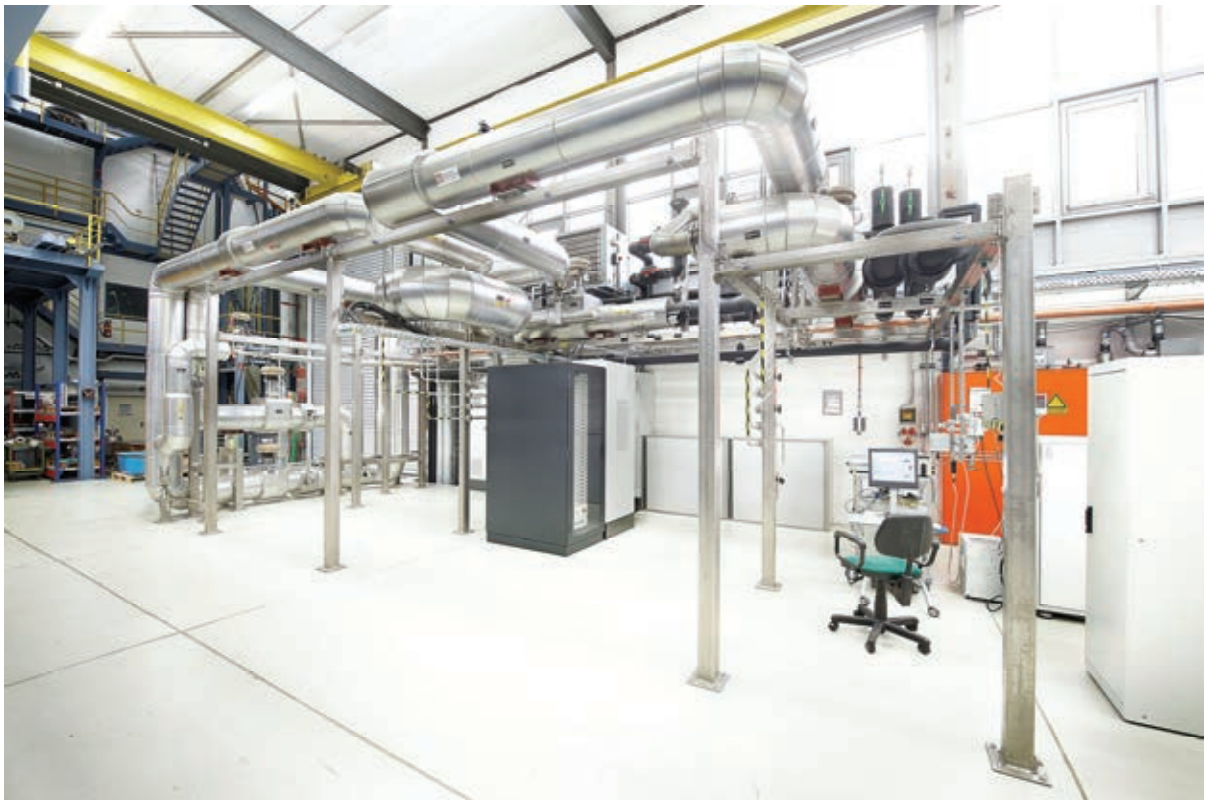
Fig. 6: Views of the HELOKA-LP facility. Top: the compressor station showing the helium compressor with two buffer vessels. Bottom: The test facility where the HFTM will be integrated, showing the piping, the switch cabinets for data acquisition and 36 power supplies and the test stand for gas analysis.
