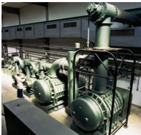
Fig. 2: 8-ary vacuum pump station of the 300 W@1.8 K-refrigerator.
