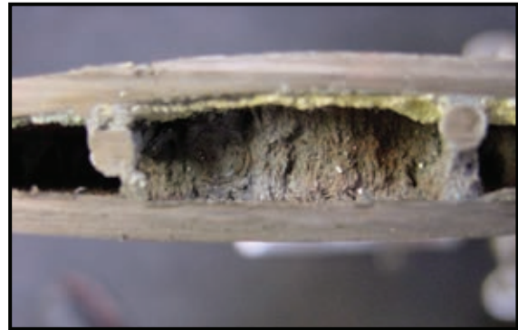
Fig. 7: View into plugged pumping channel of PICOLO loop due to precipitate collection
