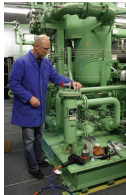
Fig. 4: Filter changes at two oil-sealed screw compressors for helium.
