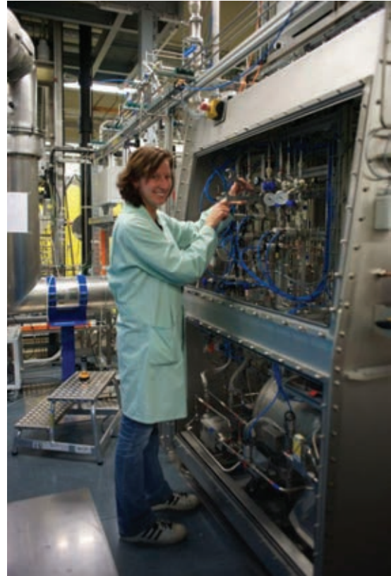
Part of TRENTA facility.
