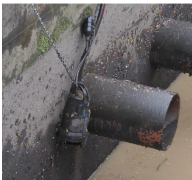
Figure 1 Submerged pump in the inlet of a stormwater sedimentation tank
