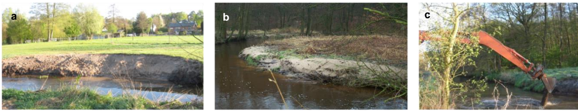
Figure 3 (a) Bank erosion (photo: Deckwerth, ULV Este). (b) Sedimentation (photo: Gumz, Landkreis Harburg). (c) Resulting maintenance measures at the Este River (photo: Deckwerth, ULV Este)
