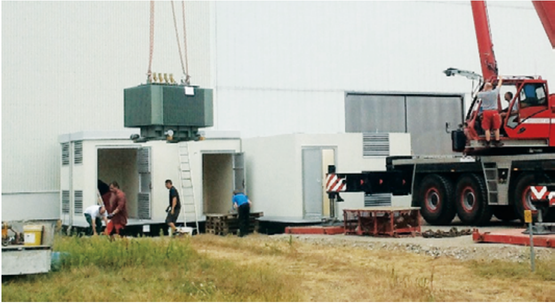
Fig. 1: installation of a new 2 MVA Transformer for the HELOKA power supply upgrade.
