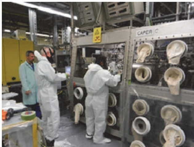
Intervention in CAPER C to install new equipment for R&D on highly tritiated water.
