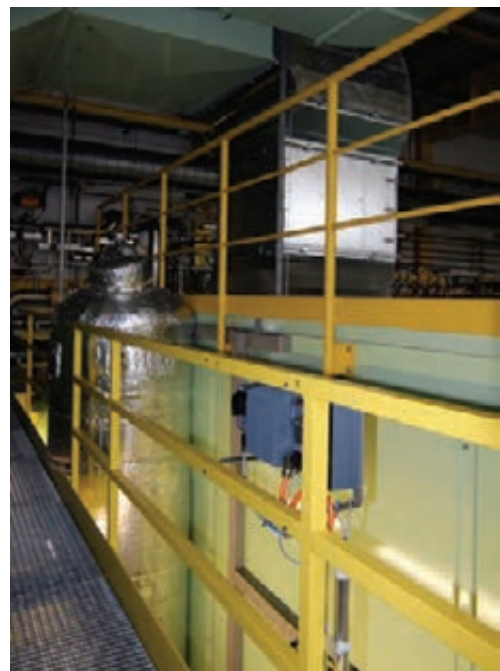
Fig. 4: New design and reconstruction of the ventilation system of the noise cancelling box.
