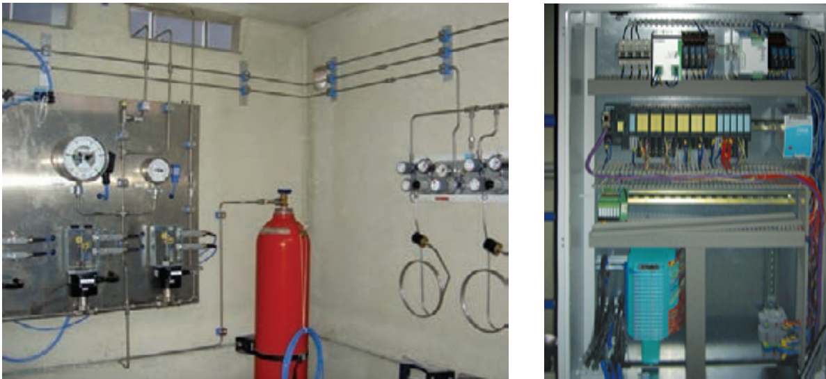
Fig. 5: The hydrogen interlock system with the intermediate storage (left) and the safety relevant control system (right).
