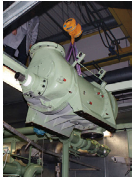
Fig. 3: Revision of the screw compressors of the 2 kW-He-refrigerator.
