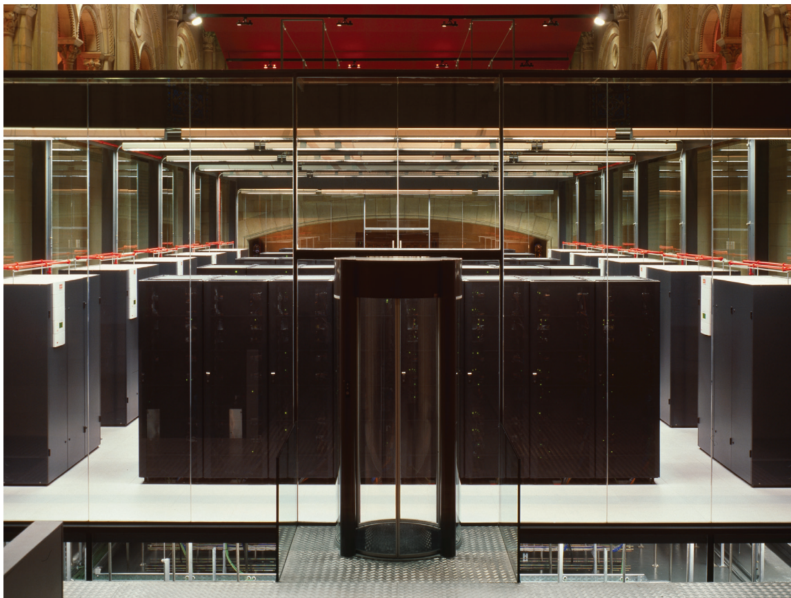
The supercomputer MareNostrum, located in an old chapel built in 1920, is one of the fastest supercomputers in the world and the main resource of Barcelona Supercomputing Center
