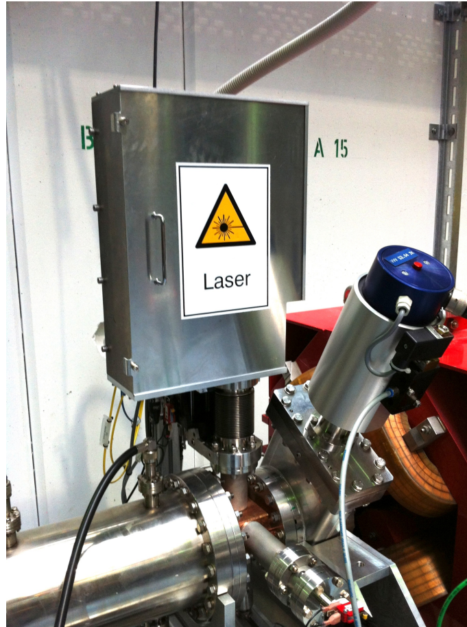
Figure 5.12: Photograph of the EO-Monitor after installation. It is located in Sector 3 between a stripline at the end of a long straight section (left) and a vacuum valve which is followed by a quadrupole (right).
