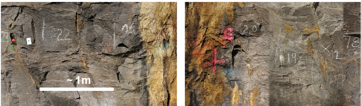
Figure 3.4: Pictures of the geological mapping of Kopf et al. (2008). From 18 - 22 m a large joint occurs which can be distinguished by a yellowish-brownish colour (joint number 24). The scale of the two pictures is almost the same, but only roughly estimated from the 1 m indicators (white dashes) in the pictures. Due to the slightly different perspectives, the images cannot be directly put together.
