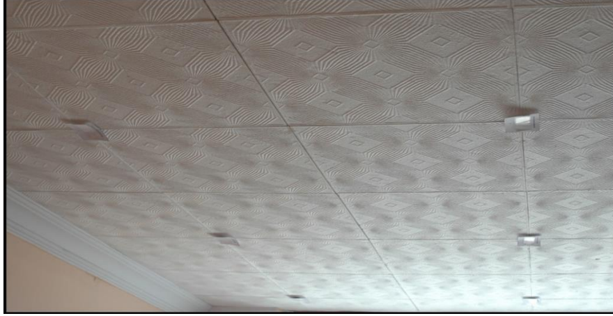
Fig. 4 Image of the room in which Model 3 has been installed
