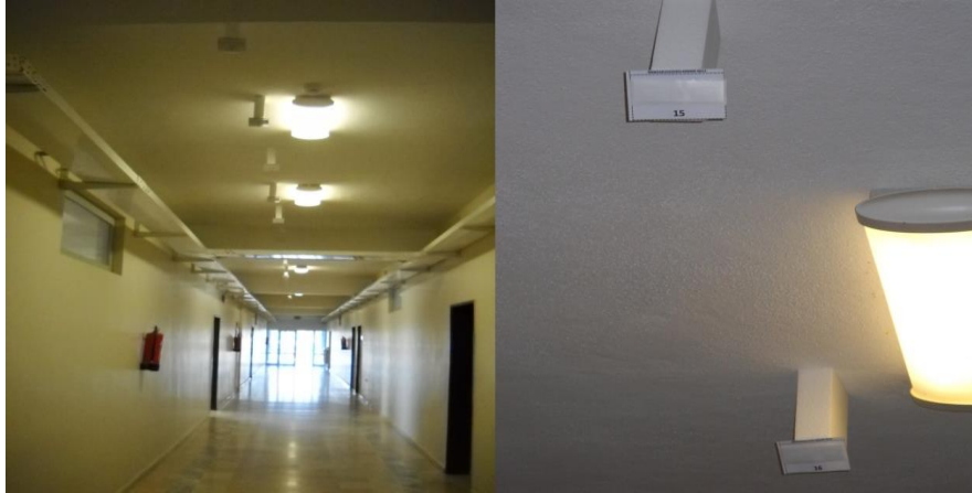
Fig. 2 Image of the corridor having tags plugged on ceiling in which Model 1 has been installed
