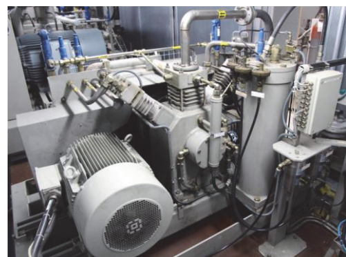
Fig. 4: Revision of the He-recovery compressor V40.
