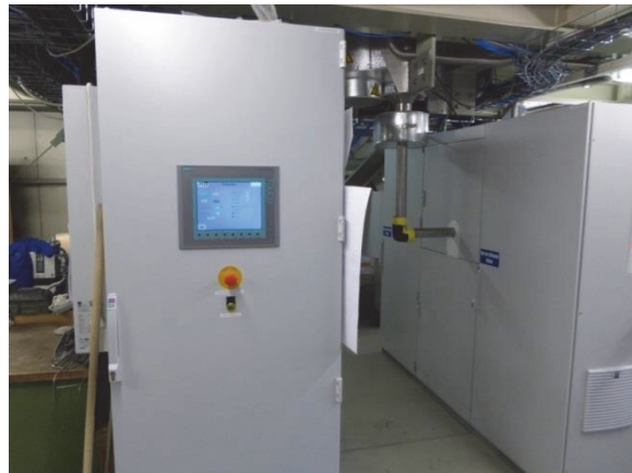
Fig. 5: Mercury vapour monitoring system and liquid ring pump housing in THESEUS (lower level).
