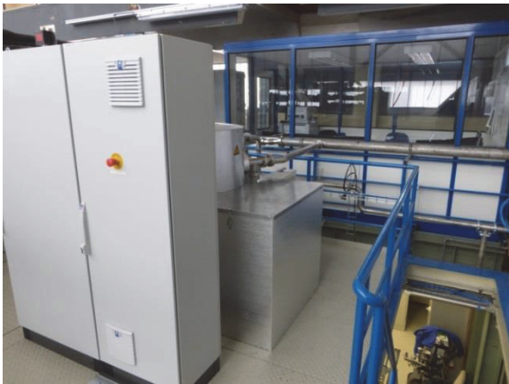
Fig. 4: Gas dosing system, dosing dome and control room in THESEUS (upper level).
