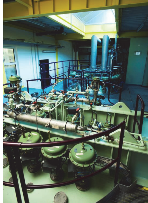
Fig. 2: Cold box and valve box of the 2 kW-He-refrigerator.
