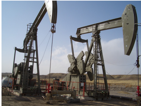
(b) Pump jacks at an oil well in the fields of Duchesne County
