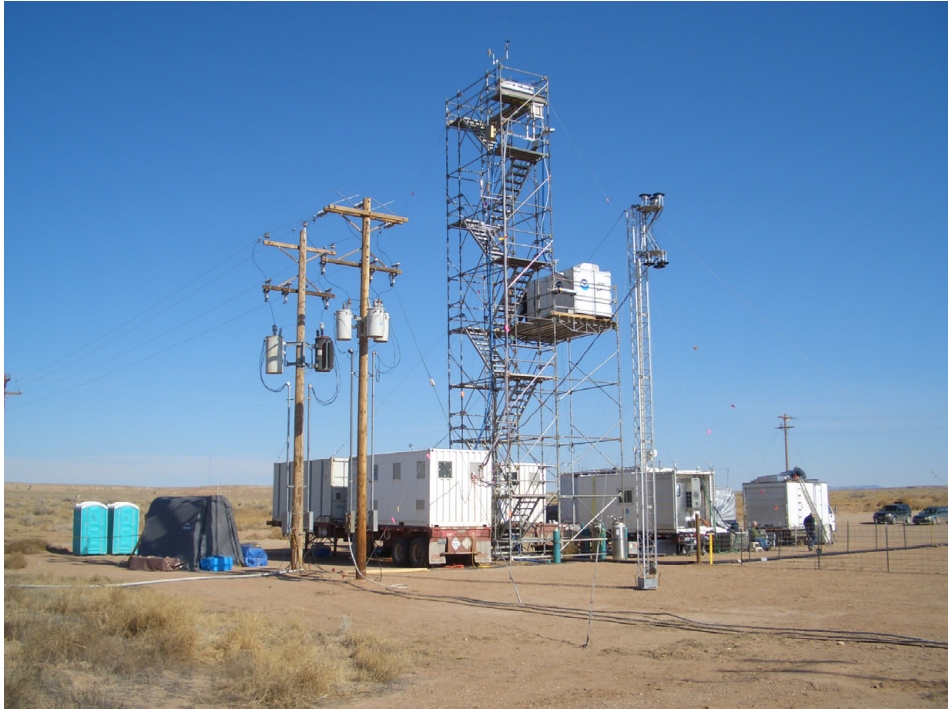
Figure F6.5: The field site Horse Pool with major part of the stationary measuring instrumentation distributed to several instrument containers, the open scaffolding and other outside equipment (like e.g. radiometer tower). The picture was taken on 4 February 2012.
