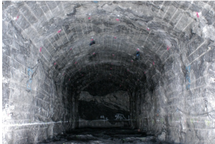
Fig. 7. Gneiss in URL Onkalo, Finland. Dark spots are water inflows on joints. Vira, 2013
