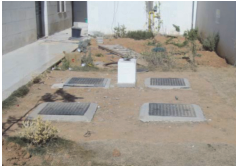
Figure 46: Modified septic tank of Eng. Akeel
