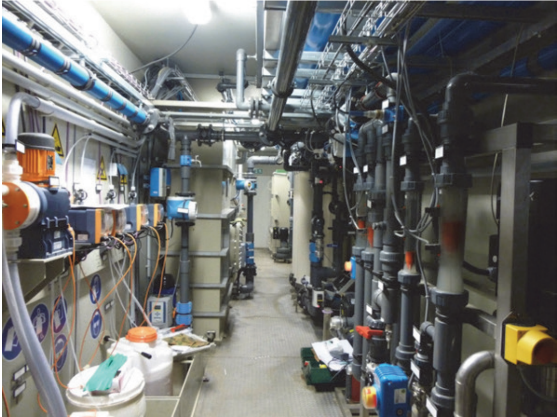
Figure 111: Pilot plant (interior of the container) in Karameh.
