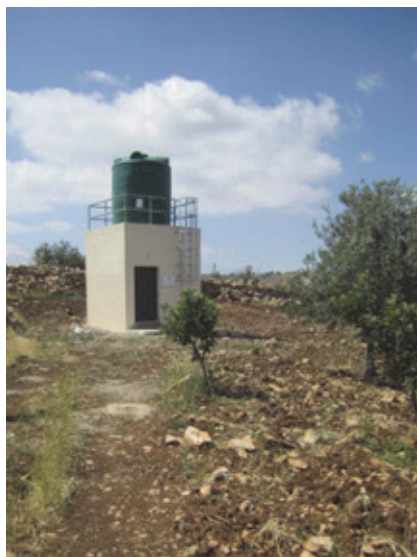
Figure 51: The Sequencing batch reactor at the nursing home, Fuheis.
