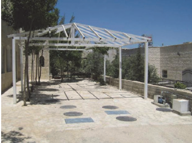
Figure 44: Modified septic tank of Mr Al Hiyari
