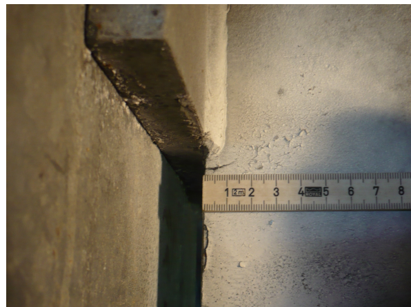
Crack caused by liquid metal embrittlement, found at the end of the half-plate weld
