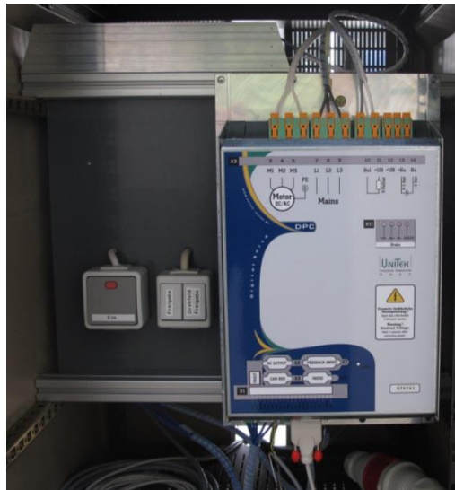
Figure 6.5: Digital servo power amplifier DPC 460 used in the setup.
