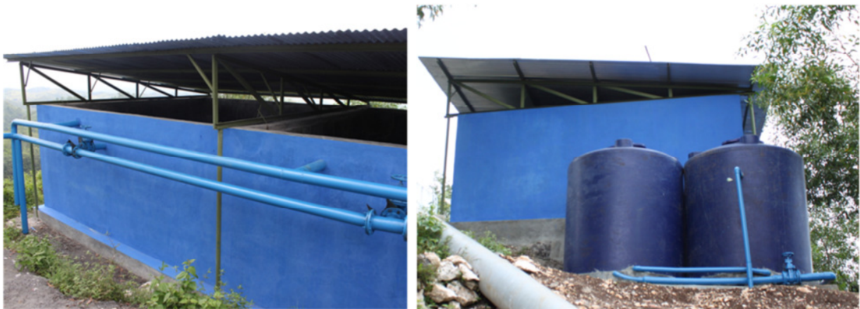
Figure 4: Sand filter installed at first reservoir following water extraction.
