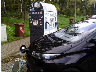
Figure 9.11.: Vandalized fast charging station at a motorway rest area [680]
