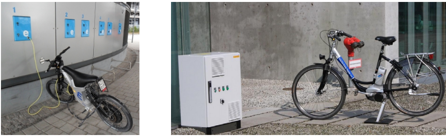
Figure 2.17.: Charging facilities for LEVs: conductive (author's photo) and inductive [122]
