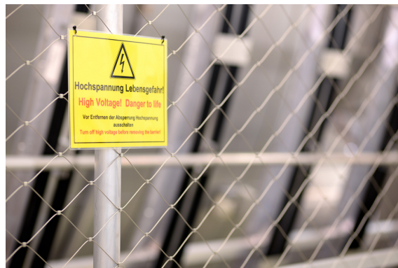
Figure 4.1: Part of the safety fence, as seen from the outside of the high voltage area. Kindly provided by Klaus Mehret.
