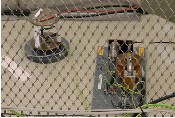
Figure 4.9: Picture of the post-regulation main parts, located at the source side of the spectrometer inside the high voltage area. On the left side of the picture the auxiliary voltage divider is seen, while the actual regulation happens with the triode-shunt on the right side. Both components are prototypes and will be upgraded for the next measurement phases, as their necessity has been proven during the second spectrometer and detector section measurement phase. Note that they are located inside the high voltage area for two reasons. For one, both are posing openly accessible high voltages and are not safe from touch. Secondly, fast regulating voltages between nodes implies their connection to be low-impedant, i.e. their connecting cables to be short.
