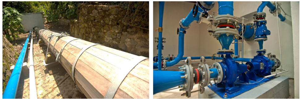
Fig. 3 Wood stave penstock (left) feeding the PAT-driven water supply system (right) of the demonstration facility
