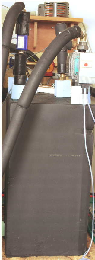
(a) Image of the adsorption chiller
