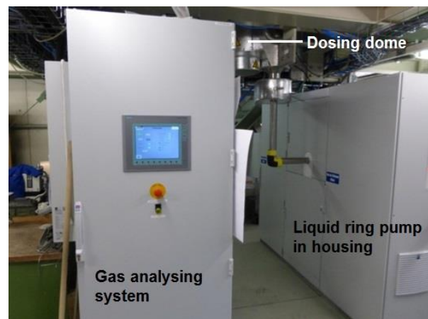
Fig. 36: Lower level: The liquid ring pump is located in the housing on the right; the connection to the dosing dome can be seen in the middle. On the left the board for the gas analysing and mercury tracking systems.
