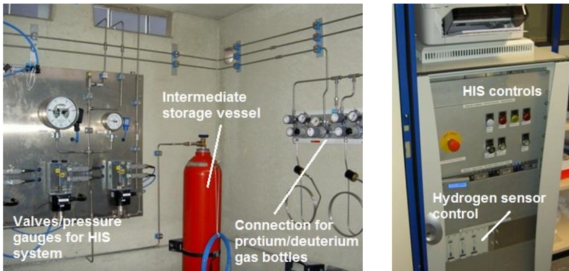
Fig. 40: The Hydrogen Interlock System (HIS): Left the installation in the gas storage and left the hard-wire controls in the control room.
