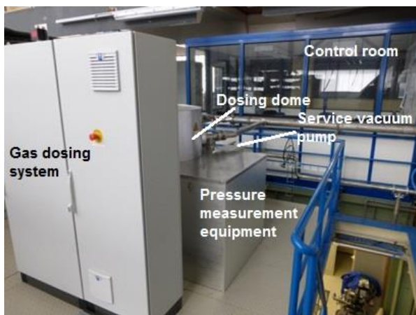
Fig. 35: Upper level of THESEUS: The control room in the background, the gas dosing system in front and the dosing dome with the box for the pressure measurement equipment in the middle.
