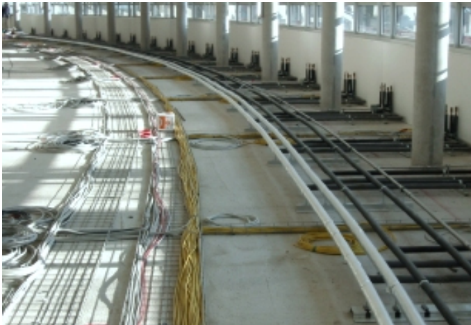
Figure 6.10: Pre-packaged materials for MEP-system installation (above); installed MEP systems (below) ( source: Digitales Bauen, Karlsruhe )
